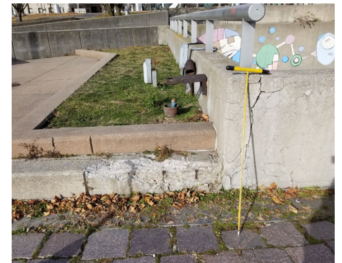
Fire and water damage to outside masonry wall in recessed area. Significant damage to painted surfaces
