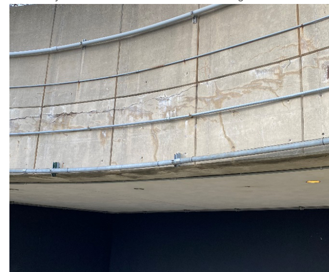
Severe horizontal cracking and significant moisture in the lower level.
