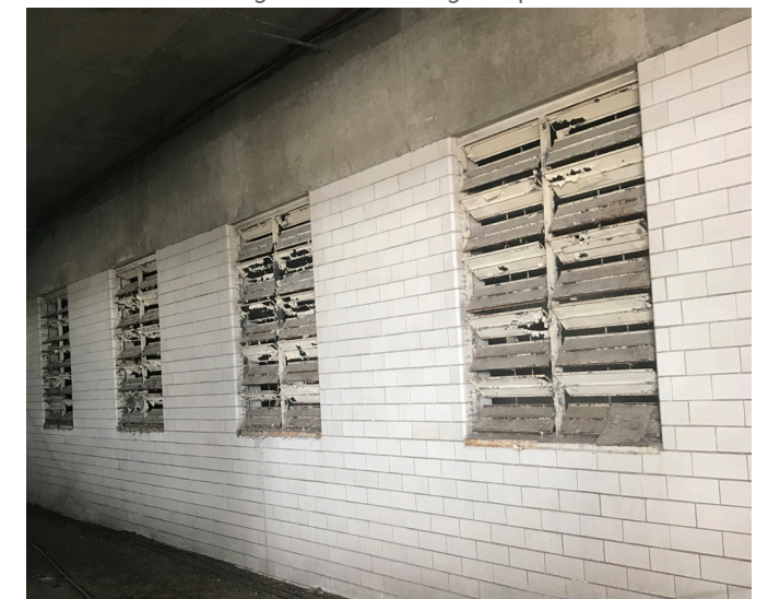
Damaged air vents in the lower level
