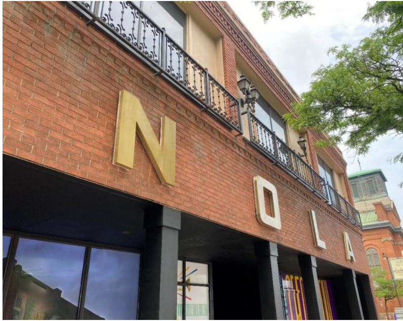
Signage installed on the front (Jefferson) façade of the building without benefit of a permit
